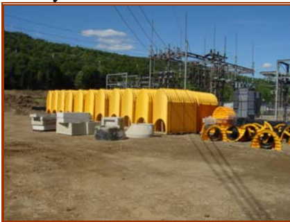
Stacked Cultec infiltration chambers
